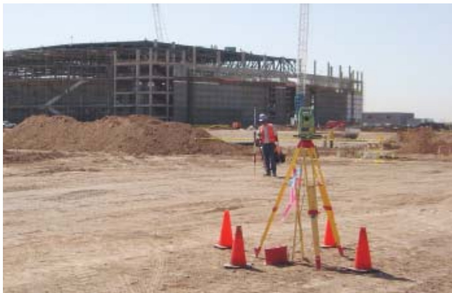
ASAM surveyors used the Leica SR530 GPS receivers and many TPS 1100 and 1103+ Professional Series robotic total stations from their inventory for the critical staking needed to complete the project.
